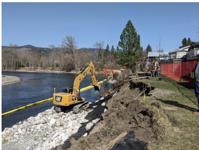
Installation of revetment on the Kettle River to curb erosion after 2018 and 2020 freshets.
